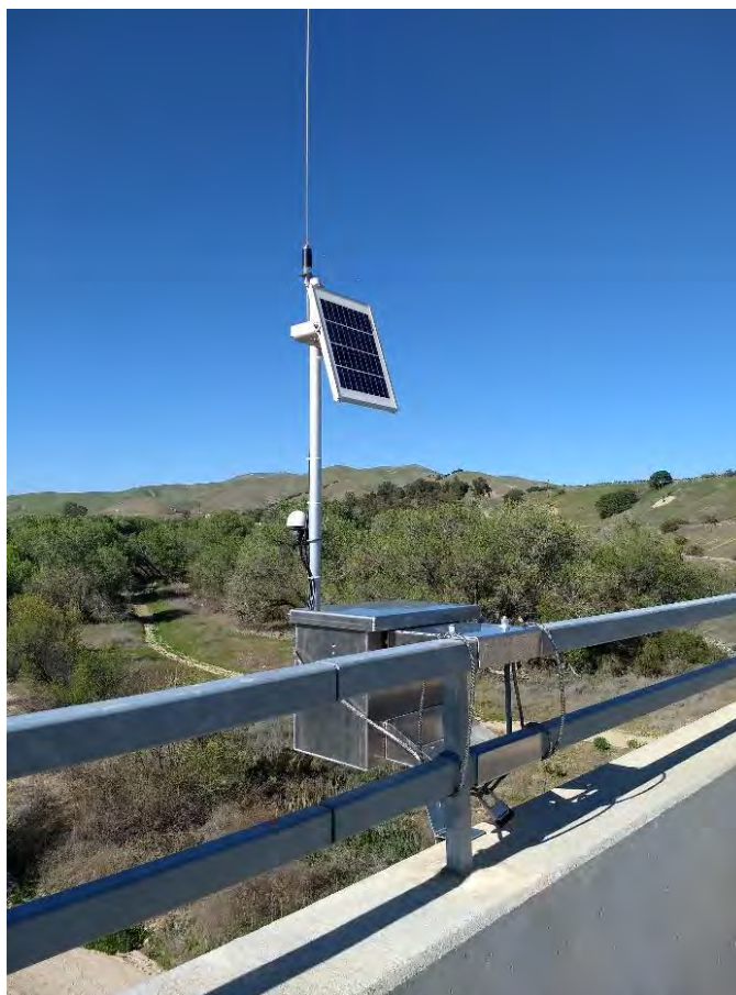
Figure 3. San Miguel (Salinas River) radar sensor stream gage installation
